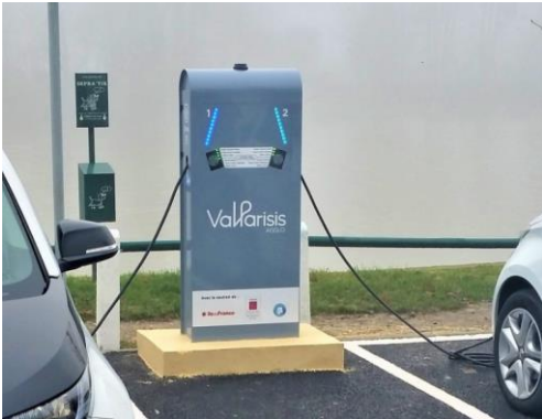
Figure 7 - Borne CITY (2x22 kW) – TOTAL EV CHARGE
